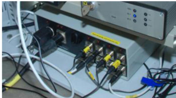
Figure 2-2: Power Distribution Box (PDB)
